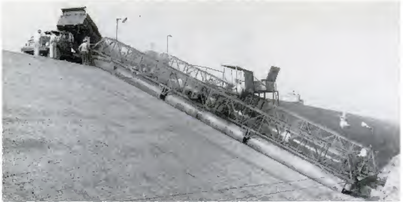
Dump truck unloads hot asphalt into side hopper of paving machine. Up to 800 tons of asphalt are laid per day
